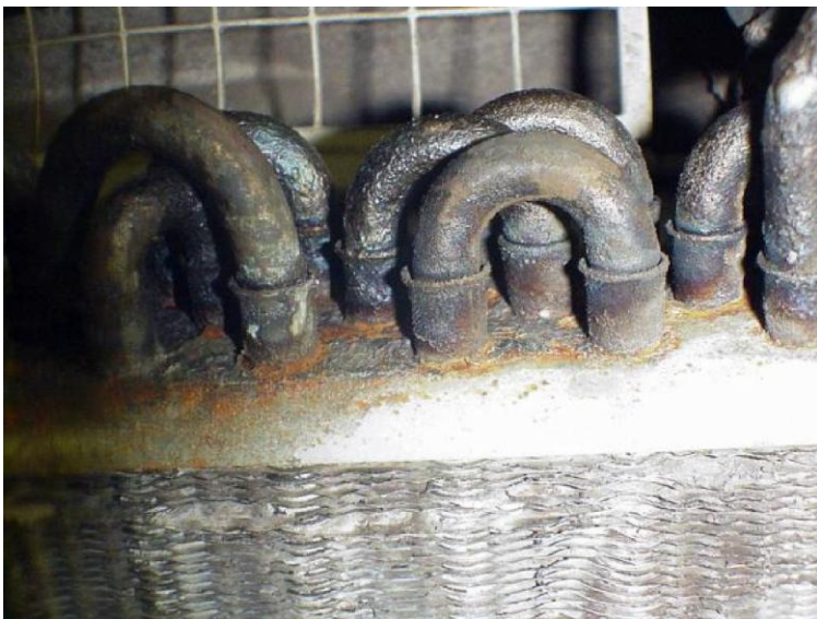
A Corroded Coil
